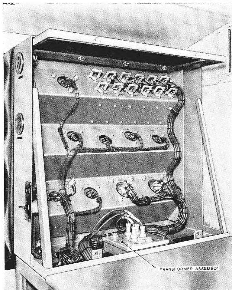
Fig. 3. Cable junction panel
