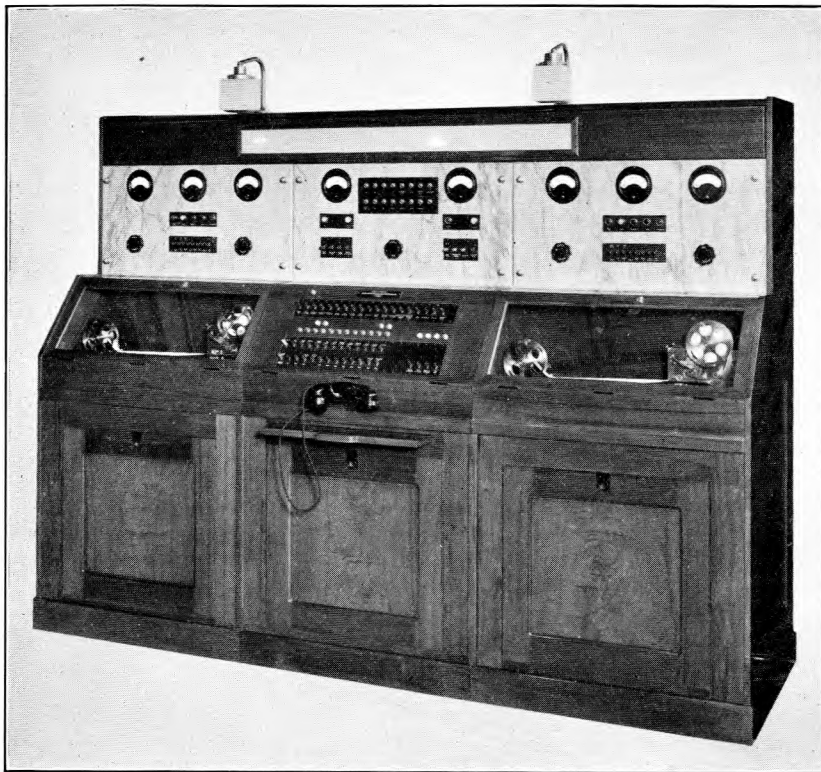
FIG. 6.—STATION EQUIPMENT AT HEADQUARTERS, LAMBETH.
