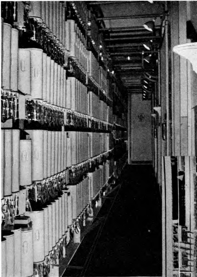
Final Selector Racks, Norte.
