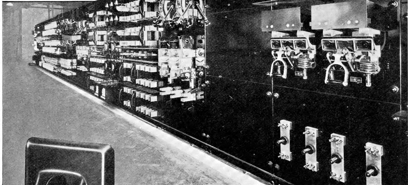
We are indebted to Messrs. William Lucy & Co. Ltd., of Oxford, the Electrical Manufacturers, and Messrs. Rashleigh, Phipps & Co. Ltd., the Electrical Contractors, for permission to publish this photograph.
