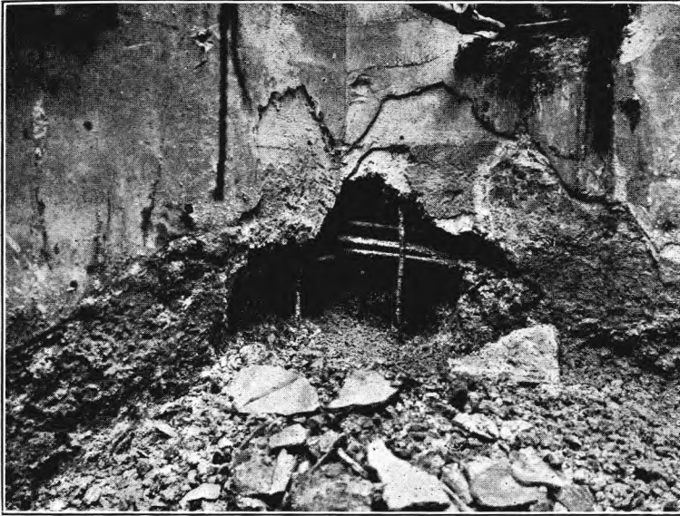
FIG. 3.—FURTHER EFFECTS OF SULPHATE CORROSION.
