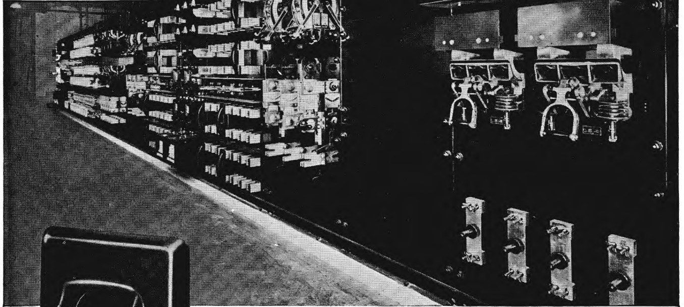
We are indebted to Messrs. William Lucy & Co. Ltd., of Oxford, the Electrical Manufacturers, and Messrs. Rashleigh, Phipps & Co. Ltd., the Electrical Contractors, for permission to publish this photograph.
