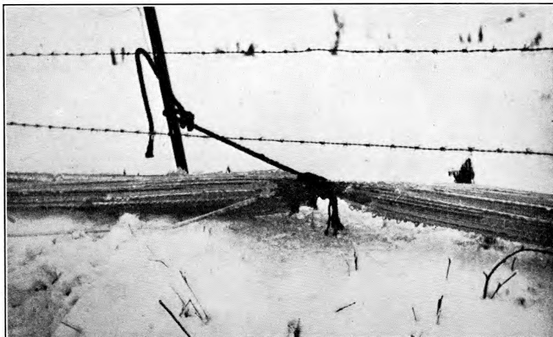
FIG. 5.—FALLEN WIRES FROZEN IN SOLID MASS ON THE OXFORD-WANTAGE ROUTE.
