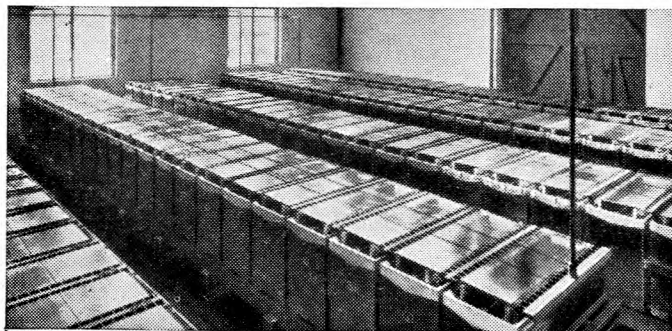
Part of the Alton Battery equipment installed at the B.B.C. Scottish Regional Transmitting Station.
