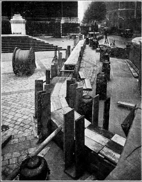
FIG. 5. TEMPORARY CABLE IN TROUGHING.
