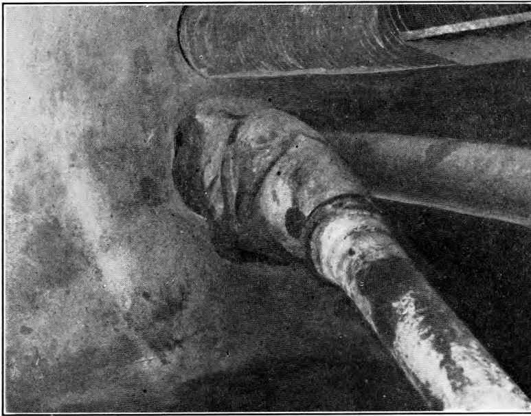
FIG. 3. DAMAGE TO CABLE JOINT AT MANHOLE DUCT ENTRY.
