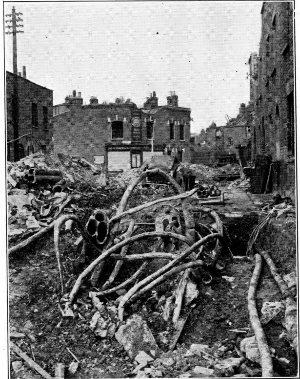
FIG. 2. DAMAGED UNDERGROUND CABLES.
