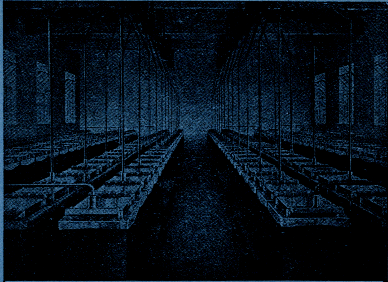
ALTON Battery of 264 DLWII Type Cells at a Corporation Electricity Works
