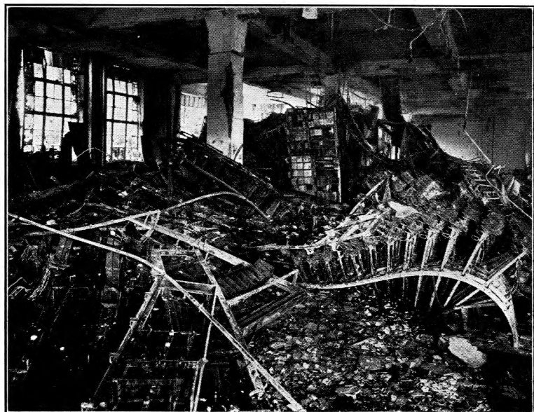
FIG. 1.—I.D.F. GENERAL VIEW OF DAMAGE.
