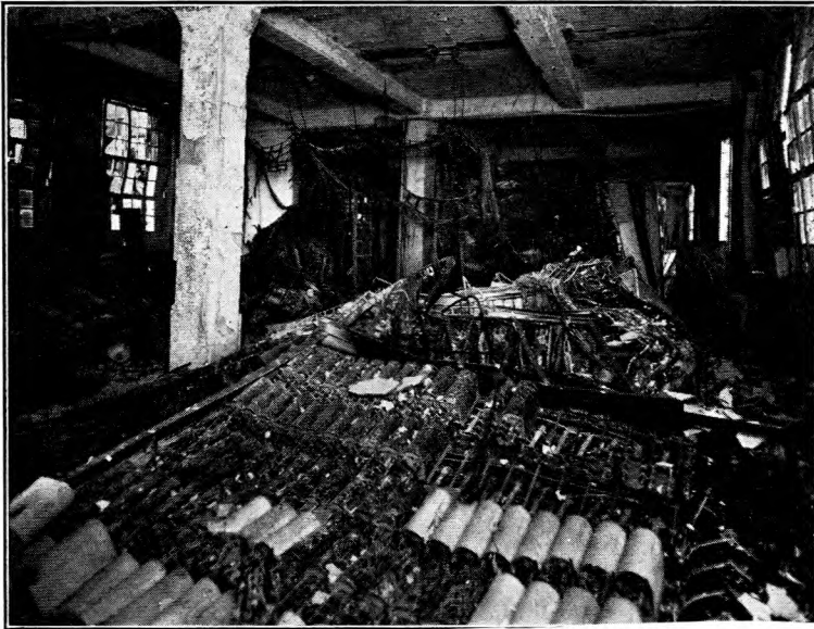
FIG. 2.—SELECTOR RACKS. THIRD FLOOR.
