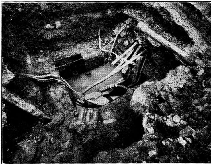
FIG. 4.—DAMAGE TO UNDERGROUND PLANT (BRIXTON, LONDON)
