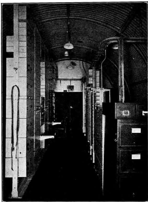
FIG. 5.—3- and 12-CIRCUIT CARRIER EQUIPMENT IN UNDERGROUND ACCOMMODATION AT CUCKMERE.
