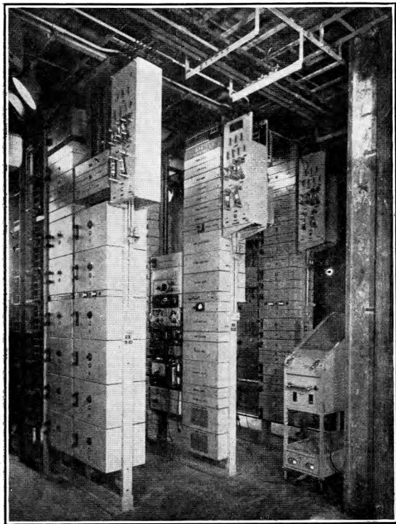
FIG. 4.—12-CHANNEL CARRIER EQUIPMENT INSTALLED IN CALAIS REPEATER STATION.
