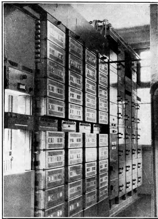
FIG. 5.—BRITISH CARRIER EQUIPMENT INSTALLED ALONGSIDE FRENCH EQUIPMENT IN AMIENS REPEATER STATION.
