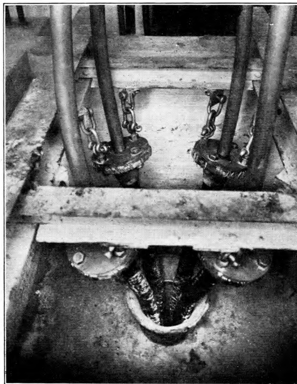
FIG. 5.—CABLE GRIPS OVER BORE TUBE.
