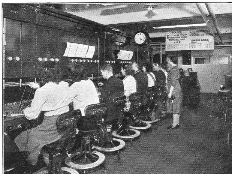
FIG. 1.—CORINTHIAN EXCHANGE—PART OF SWITCHBOARD
