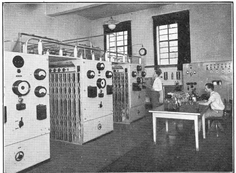
FIG. 5.—HIGH-POWER AMPLIFIER STAGE OF V.L.F. TRANSMITTER.
