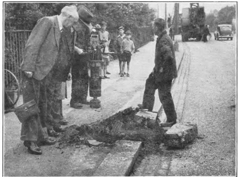
FIG. 4.—DISTURBANCE OF FOOTWAY—THE WORST CASE.
