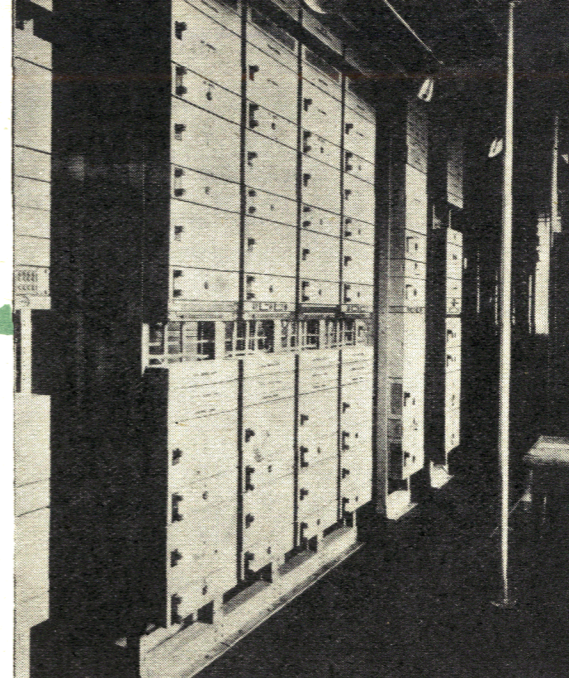
Coaxial system bays at Kidderminster.
