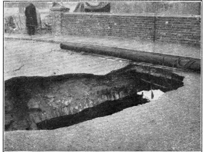
HOLE IN BRIDGE AT HADLOW, SHOWING TEMPORARY SUPPORT FOR ONE POST OFFICE CABLE.
