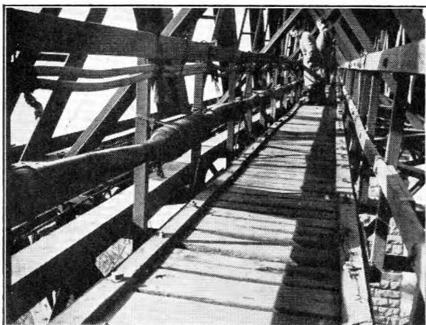
FIG. 4.—INTERRUPTION CABLE ON CATWALK.
