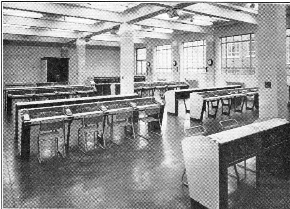
FIG. 1.—GENERAL VIEW OF THE SWITCHROOM AT THANET EXCHANGE.
