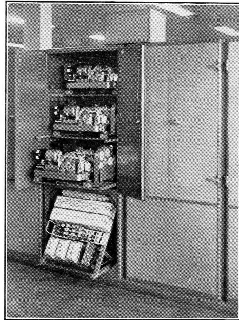
FIG. 4.—REAR VIEW OF PRINTING REPERFORATORS, SHOWING APPARATUS WITHDRAWN FOR MAINTENANCE.
