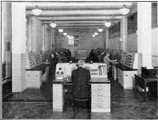
FIG. 14.—TWO SUITES OF OPERATING POSITIONS AND ASSOCIATED CONTROL POSITIONS AT THE RADIO TELEPHONY TERMINAL, BRENT.
