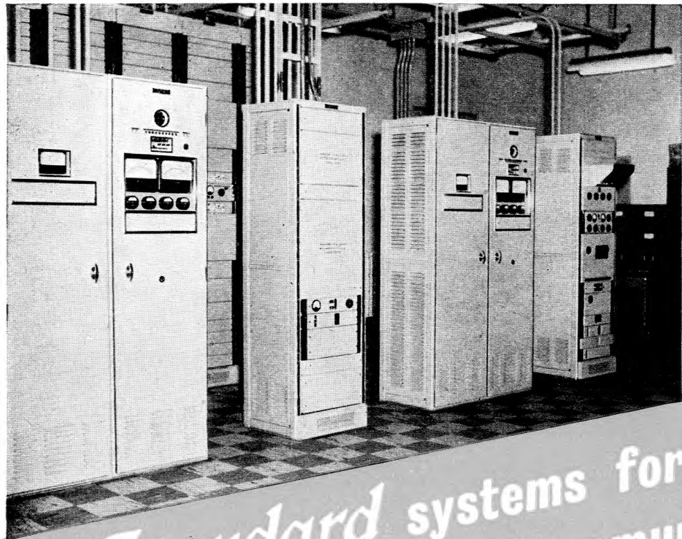
Submerged repeater power supply cubicles at Sydney Mines. Cable terminal cubicle is shown at centre.
