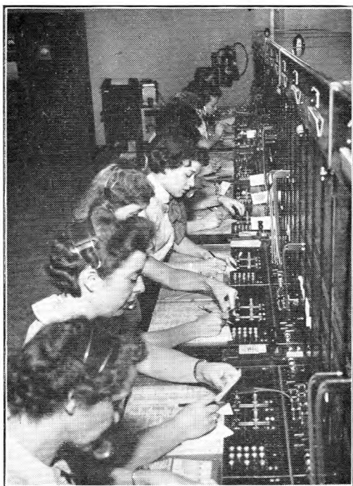
OVERSEA SWITCHBOARD IN WHITE PLAINS, NEW YORK, WHERE UNITED KINGDOM-UNITED STATES CIRCUITS TERMINATE.
