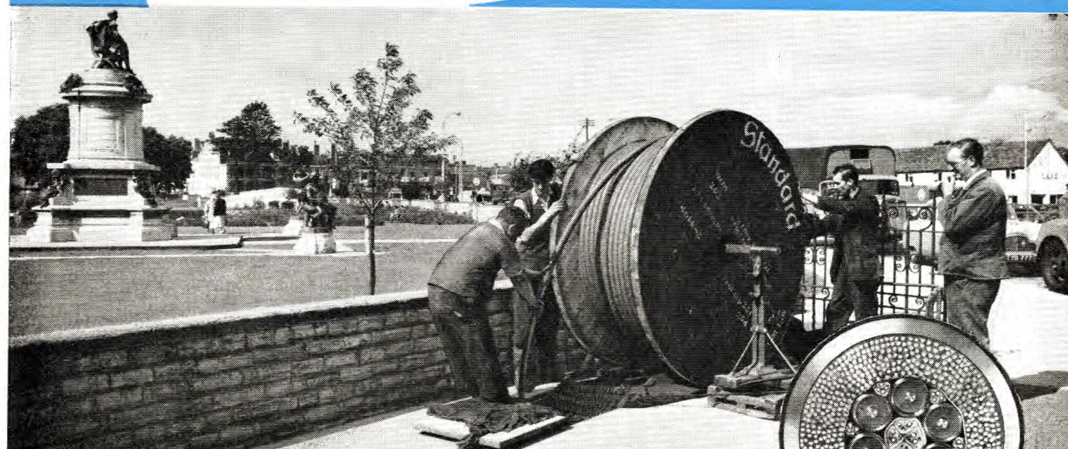
A length of the new S.T.C. coaxial cable during installation at Stratford-on-Avon.
