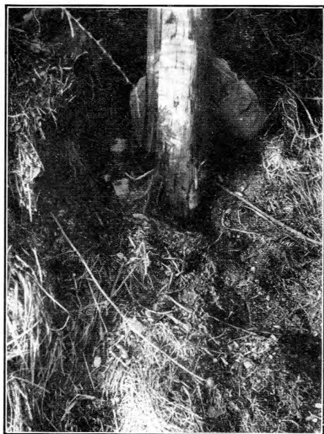
POLE DAMAGED BY LIGHTNING STRIKE.
