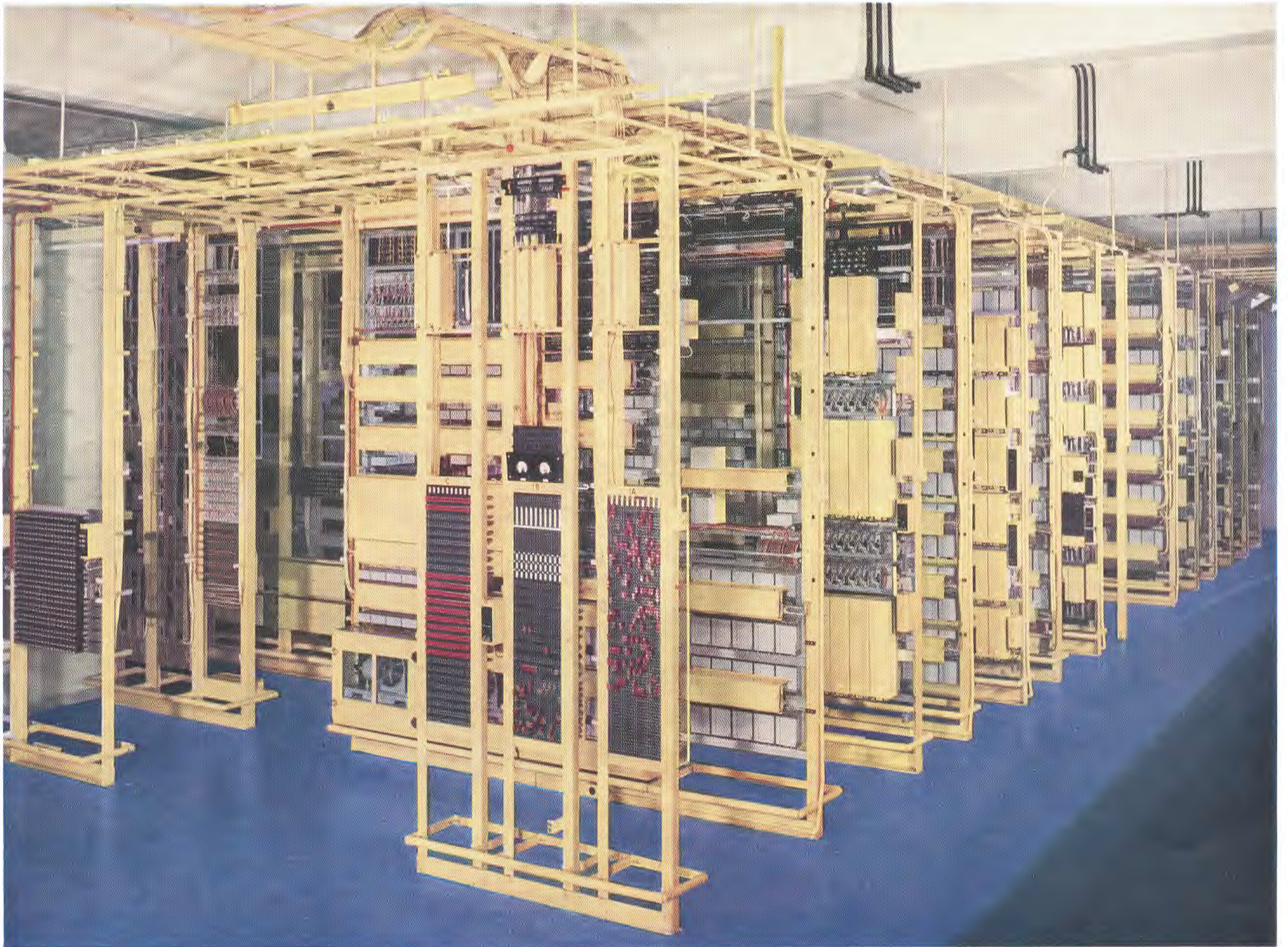
FIG. 2—THE LONDON (SHOREDITCH) AUTOMATIC TELEX EXCHANGE
