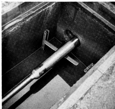
FIG. 9—EFFECT OF CABLE CREEPAGE: JOINT JAMMED IN DUCT-MOUTH
