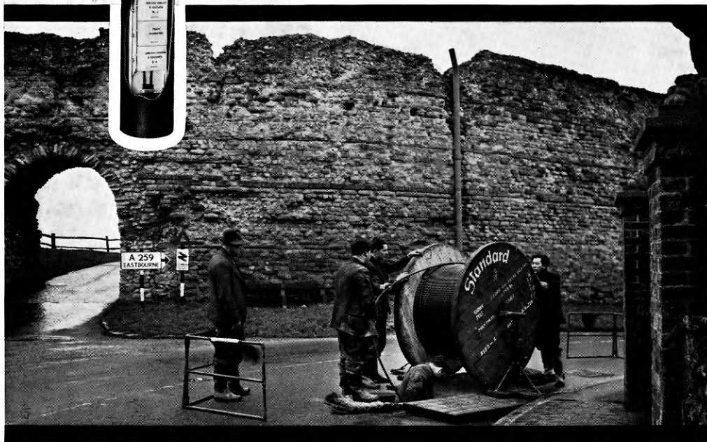
S.T.C. all-transistor buried repeater
