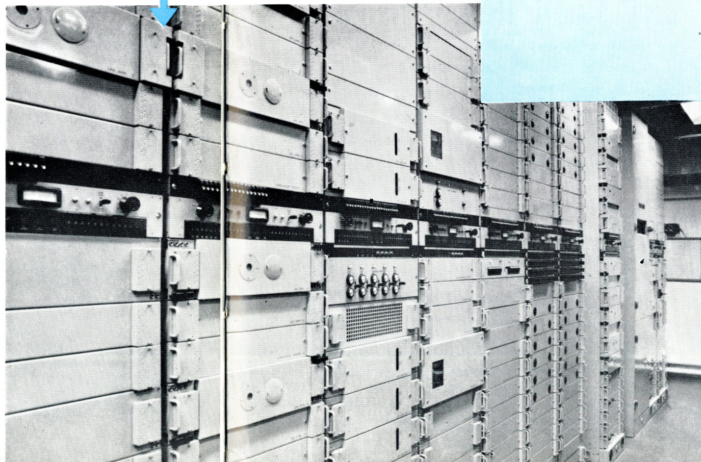
Suite of A.T.E. baysides at the Middlesbrough terminal station
