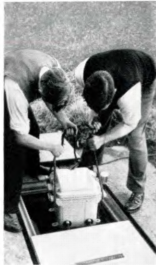
A complete 600 channel four tube repeater
