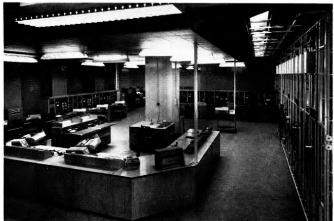
In the foreground are maintenance-control positions. FIG. 5—GENERAL VIEW OF TEST ROOM
