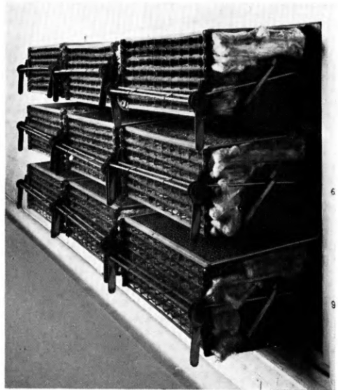
FIG. 2—TYPICAL TELEPHONE EXCHANGE PLENUM VENTILATION SYSTEM—VIEW OF FILTER
