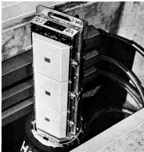
FIG. 1.—DEPENDENT REPEATER EQUIPMENT IN RAISED POSITION
