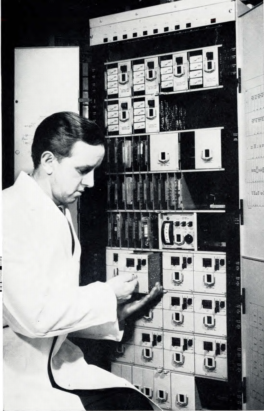
Typical Type C12G terminal rackside
