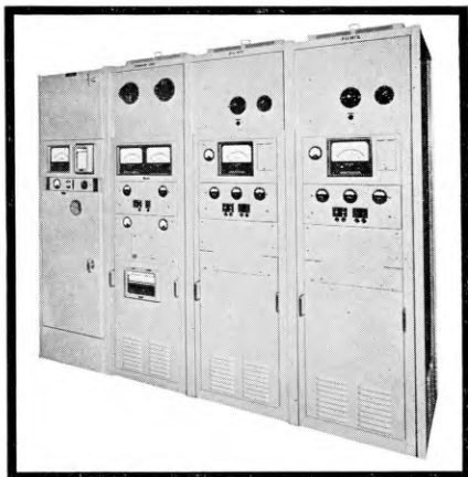
Transductor controlled submerged repeater power feeding equipment with two power units.
