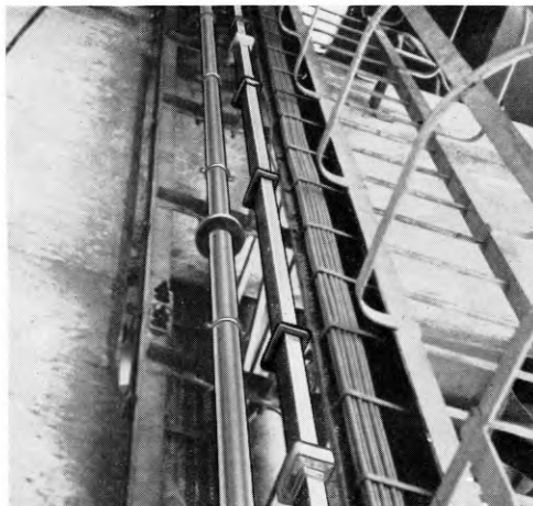
FIG. 4—THE VERTICAL HELIUM PIPE, AND THE WAVEGUIDE CARRYING THE AMPLIFIED SIGNAL FROM THE MASER
