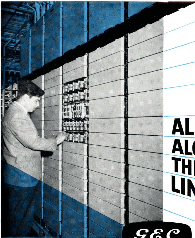
Type 56 transistored channel equipment at Faraday Building.
