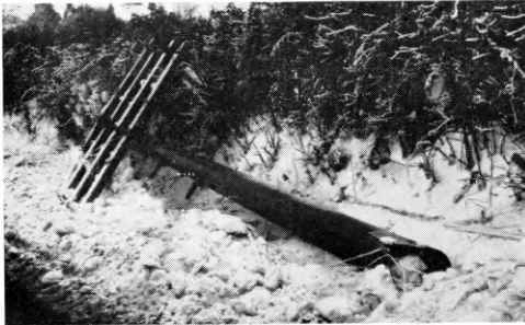
ONE OF THE COLLAPSED POLES
