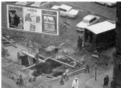
DAMAGE CAUSED BY THE BURST HYDRAULIC WATER MAIN
