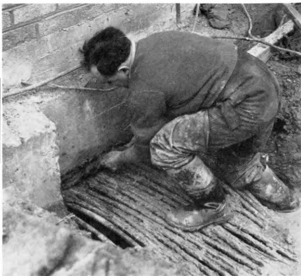
24½" diameter cables passing through duct measuring 36" × 18" × 9" which is completely filled with DENSO MASTIC.
