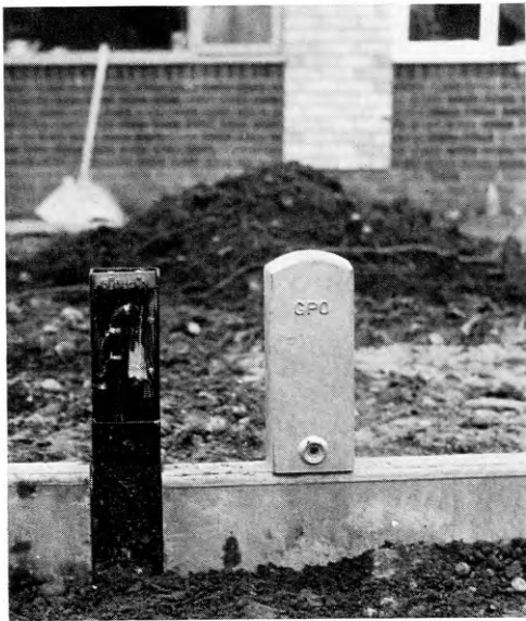
ABOVE-GROUND JOINTING POST
