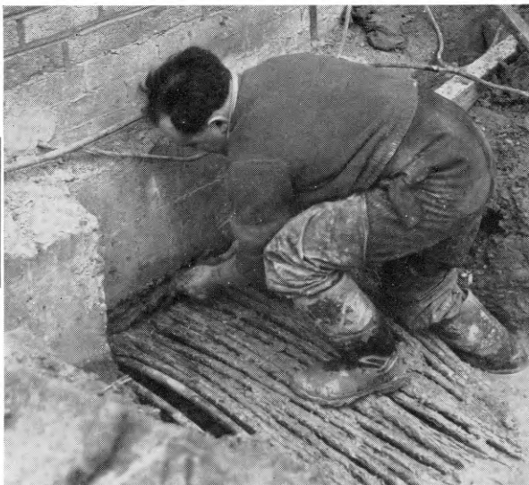
24 1/2" diameter cables passing through duct measuring 36" x 18" x 9" which is completely filled with DENSO MASTIC.
