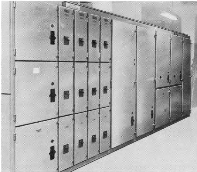
FIG. 4—PLANT NO. 1 AUTOMATIC CONTROL AND DISTRIBUTION CUBICLE
