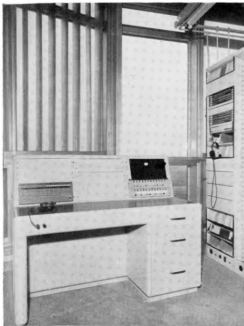
FIG. 19—ALARM AND CONTROL EQUIPMENT, FLOOR B5
