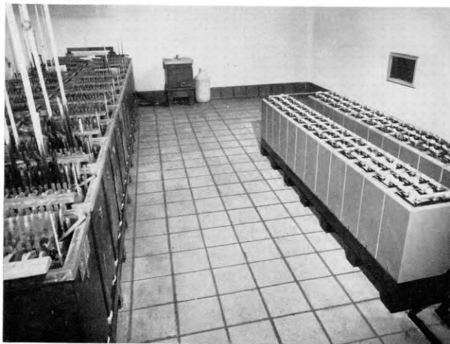
Wooden laths, inserted to prevent contact between distorted positive plates and the negative plates can be seen in the old battery on the left-hand side
