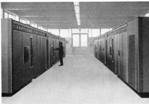
FIG. 3.—SIX OF THE 30 kW FIXED-SERVICE TRANSMITTERS
