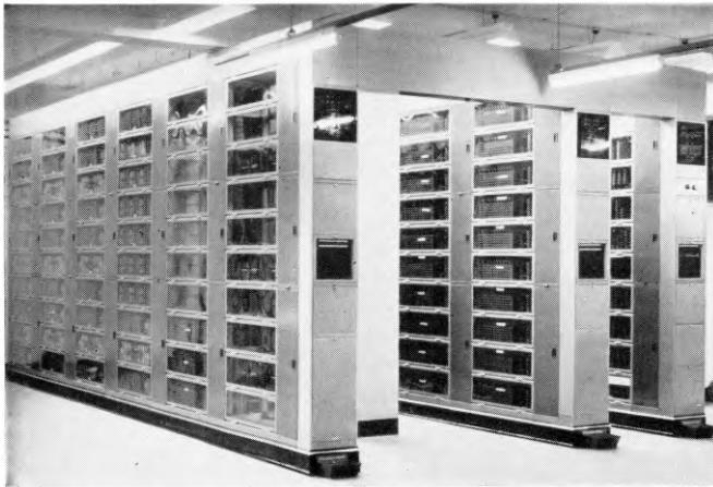
FIG. 1—5005-CROSSBAR INTERCONTINENTAL EXCHANGE INSTALLED IN SYDNEY, AUSTRALIA, FOR TERMINATION OF COMPAC CABLE
