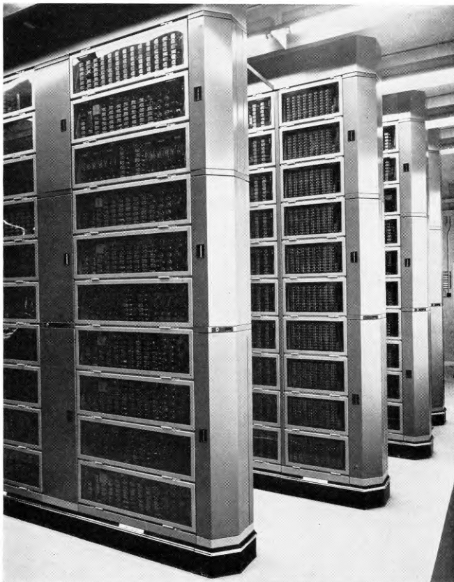
FIG. 9—GENERAL VIEW OF BROUGHTON EXCHANGE
