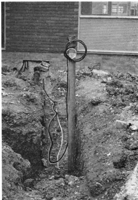
FIG. 3—LEAD-IN CABLE AND EARTH WIRE LAID BY BUILDER IN WATER-PIPE SERVICE TRENCH
