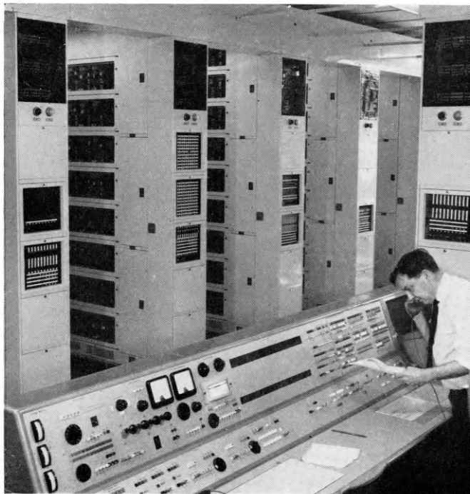
FIG. 1—EQUIPMENT RACKS AND TEST CONSOLE
