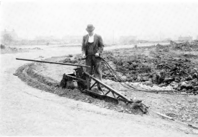
FIG. 5—POST OFFICE FOOTPATH CABLES BEING LAID BY MOLEPLOUGH BEFORE BUILDING MATERIALS ARE DEPOSITED ON THE FOOTPATH
