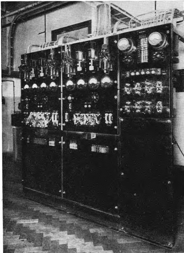
FIG. 12.—STANDARD L.T., H.T., AND 80 + 80V POWER SWITCHBOARDS FOR M.C.V.F. TERMINALS.
